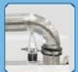
stainless steel construction & piping
